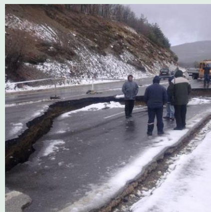
Landslide on the road M5 Resen-Bitola
